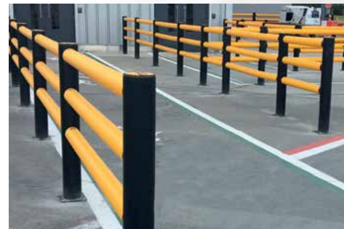
Pedestrian 3 Rail and Swing Gate
