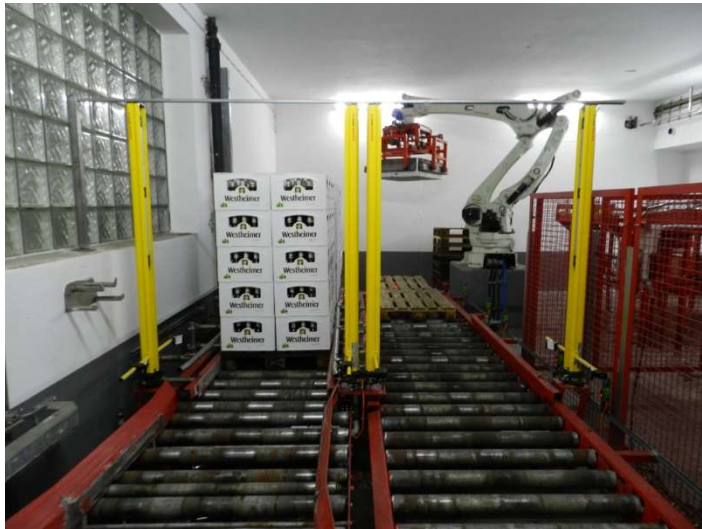
Full flexibility: The system can be adapted to new productions in the shortest possible time.
