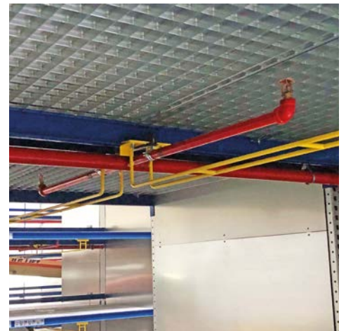
Picture caption: a sprinkler head is featured on every level and protected by a customized sprinkler guard. The sprinkler head is centered in every storage compartment for maximum efficiency.
