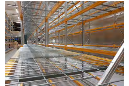
5 SHELVES Our sturdy shelves are made from steel mesh, which allows light as well as water from sprinklers to penetrate.
