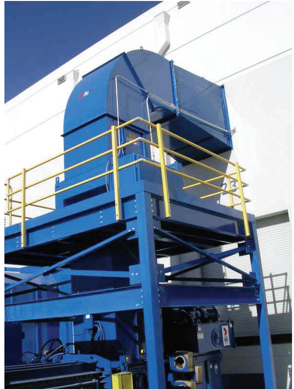
A BloApCo top feed shredder with a four side work platform mounted over an inline horizontal baler. In this installation the shredder and baler are outside the building to maximize space in the plant.
