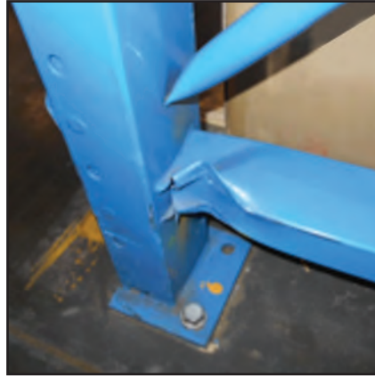
Roll formed closed tube horizontal strut damage
