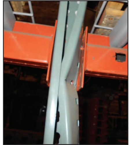
Damage behind beam connector
