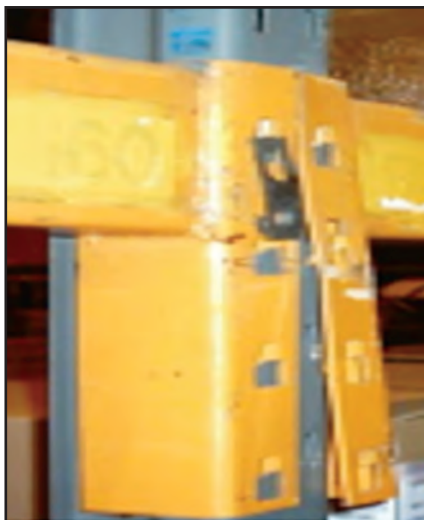
Disengaged beam end plate
