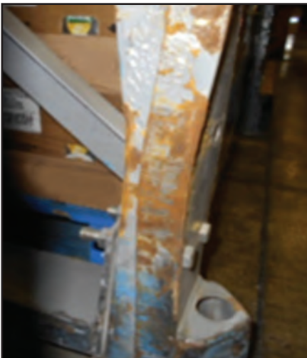
Structural column damage
