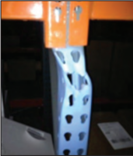
Damage under beam level
