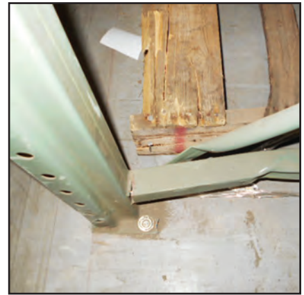
Broken strut connection
