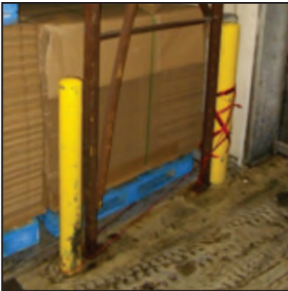
Missing horizontal struts
