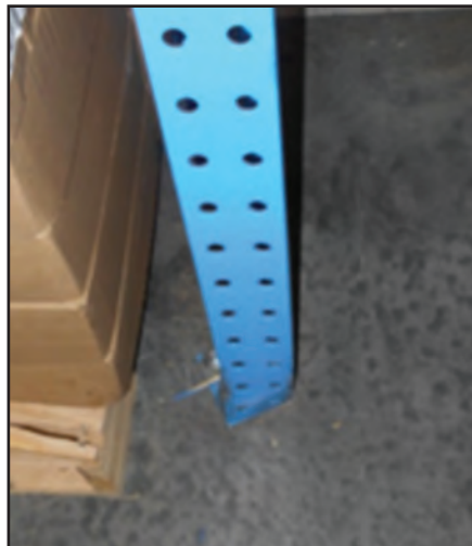
Structural column damage
