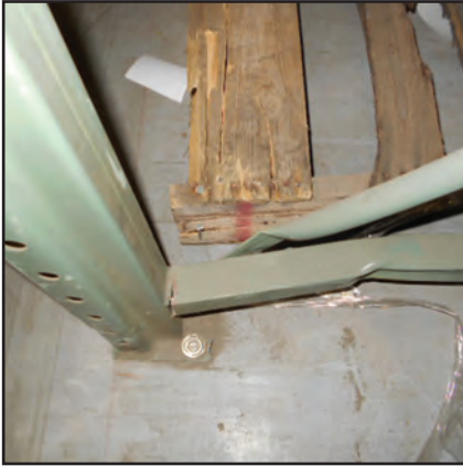
Roll formed horizontal strut damage
