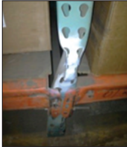
Damage above beam level
