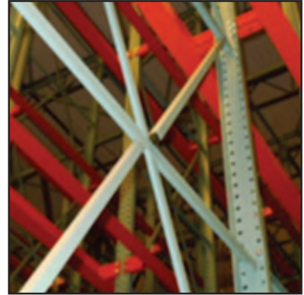
Broken diagonal weld
