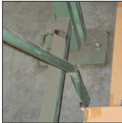
Ripped / torn horizontal and diagonal
