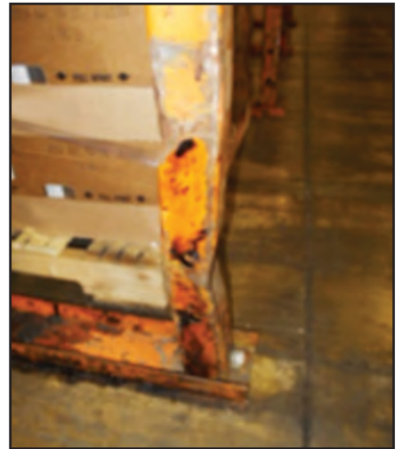
Closed tube damage
