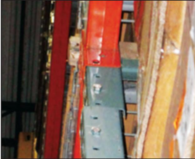
Improper splice installation
