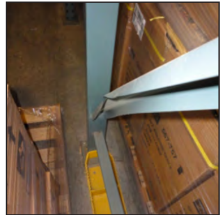
Damaged roll form diagonal
