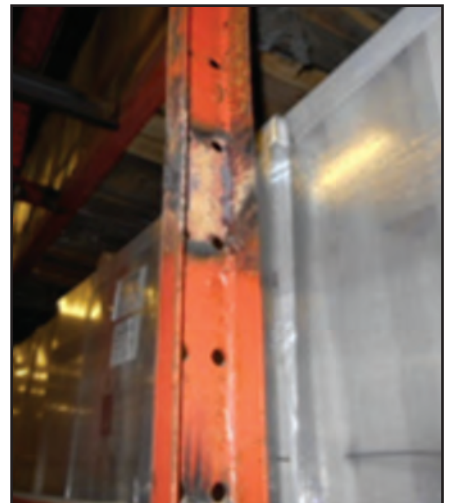
Structural column damage
