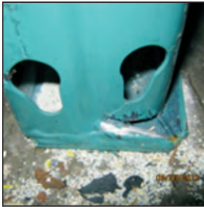
Torn footplate weld
