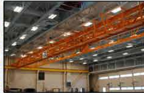
7.5 Ton 137' Span Truss Crane
