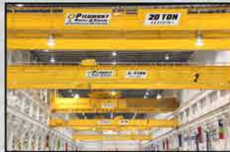
20, 30 and 250 Ton Cranes
