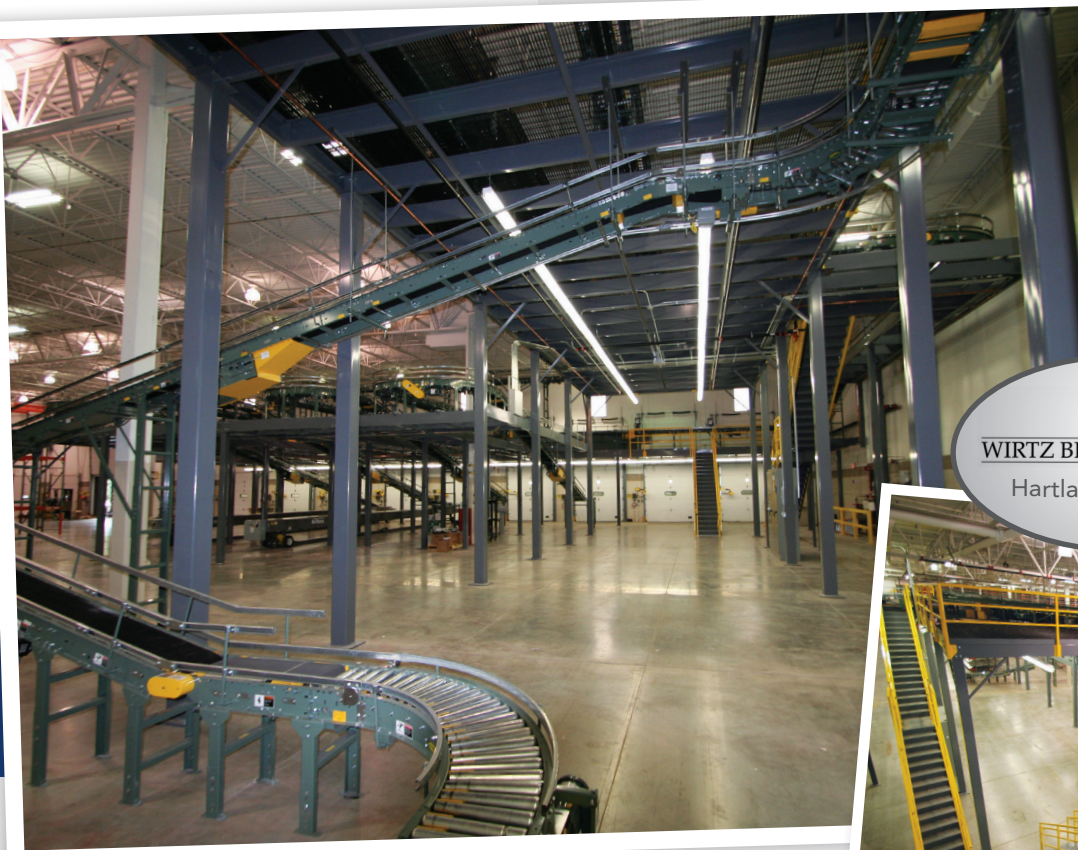
Custom designed Cubic Designs tri-level mezzanine supports multi-level conveyor system and heavy product loads.
