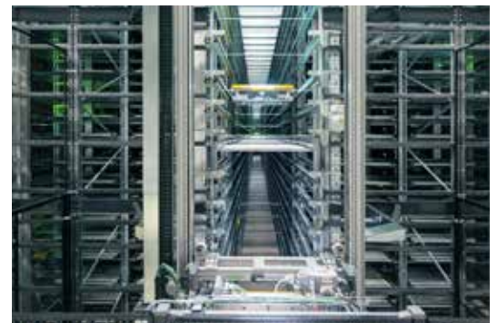
2 | The three-aisle GEBHARDT StoreBiter® One-Level-Shuttle (OLS) warehouse, realised as a Roaming+ concept with a total of 15 OLS, achieves 630 double cycles per hour.
