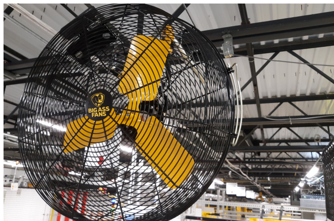
AirEye fans in testing locations on the 4th floor.
