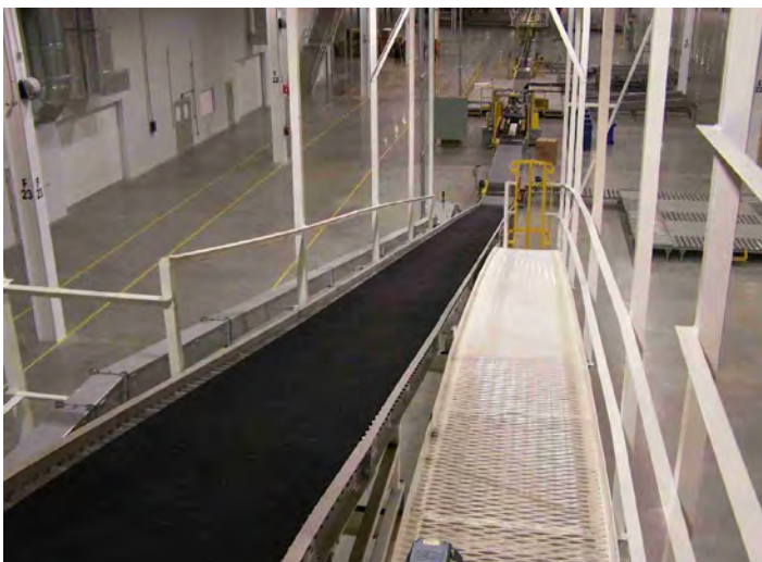
Belt Conveyors are used extensively for moving product to different elevations. This moves appliances from assembly to shipping.
