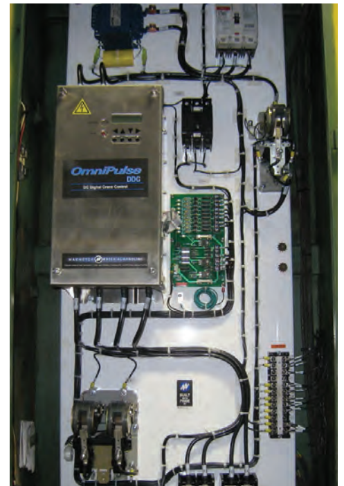
UPDATED DC Crane Control
