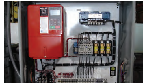
Upgrade of Above Control Package
