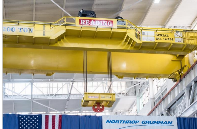
Reading Crane and Engineering Co. installed 200-ton crane with two 100-ton R&M Materials Handling, Inc. hoists at a Rhoads Industries facility.
