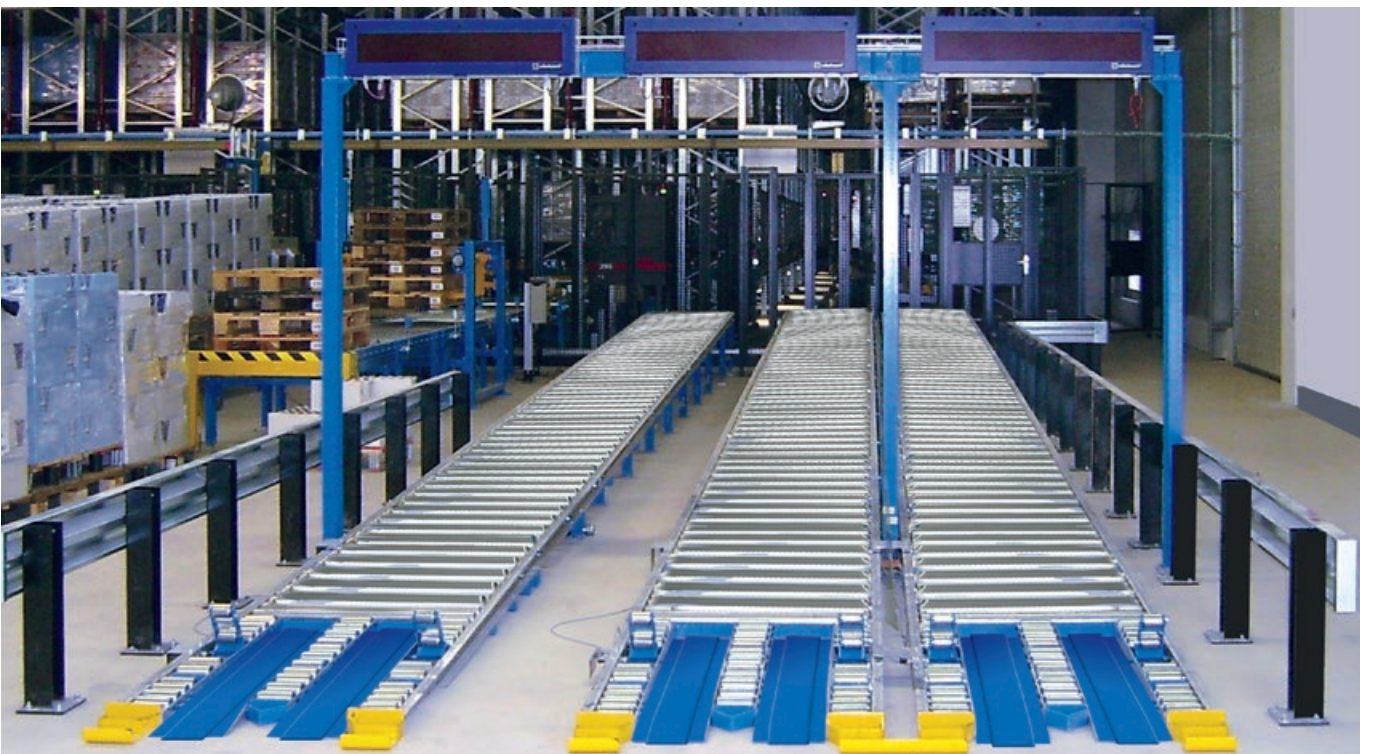
Shipping track with reinforced removal station
