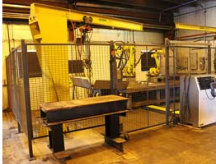
WireCrafters Machine Guarding around automated robotic welder.
