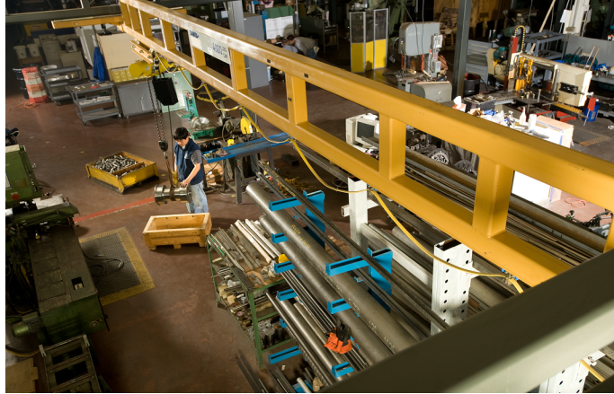
The 4,000-pound capacity bridge reaches many workstations in the facility
