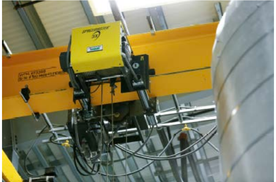
Class I, Division II Spacemaster EX hoist in the turbine room.
