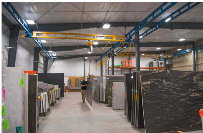
An overhead workstation crane is used by Morningstar Stone and Tile of Topsham, ME, to move stone slabs in and out of inventory. Two systems were installed, one with a motorized bridge. The previously used tow motor required two employees. Now one can do the job. Management describes the crane system as safer and more productive. Photo courtesy of Gorbel.
