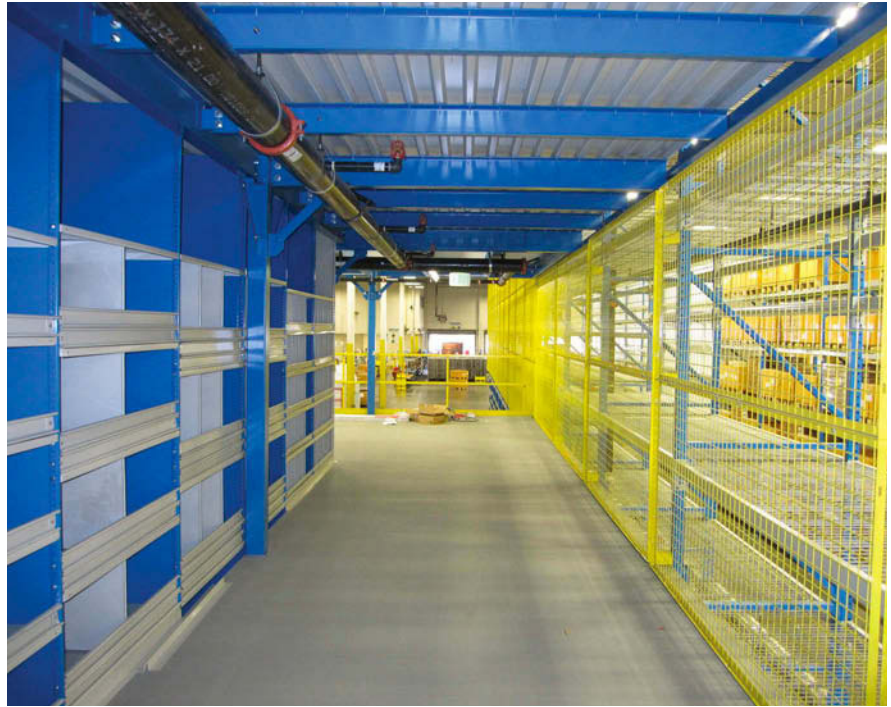
Full height rack safety panels are used to protect a pedestrian traffic aisle.
