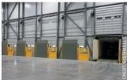
When unloading/loading at a refrigerated facility, keeping only the active door open helps with the loss of cold air during this process.
