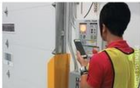
With modern technology, integrated control panels can be set up with sequenced operations.
