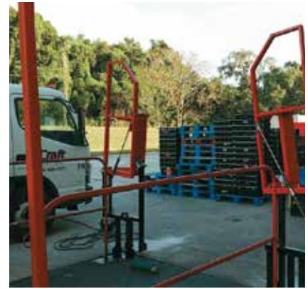
PHOTOS: MEZZANINE SAFETY-GATES
