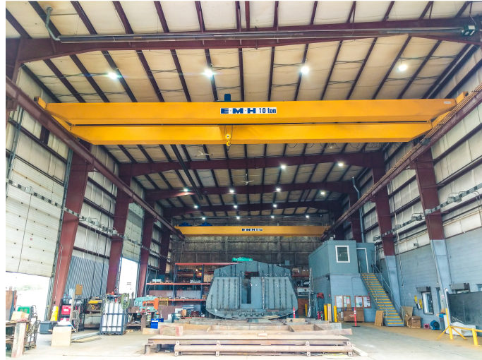
Two independently operated 5-ton lifts give the EMH overhead crane installation a combined capacity of 10 tons.
