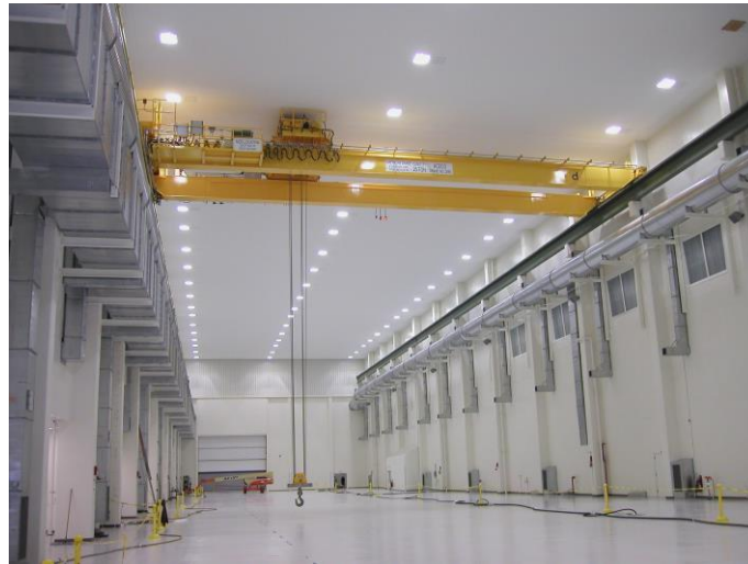
25 Ton Running Double Girder Crane
