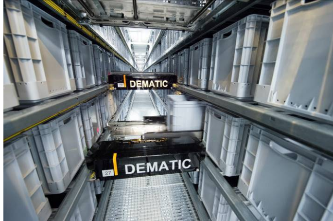
Inventory from the Multishuttle automated storage & retrieval system is transferred to the goods-to-person workstation.
