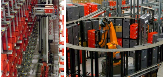
Photo: Miniload AS/RS Crane and Robot Cell
